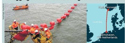
CABLE GUY: The NorNed project took four years to complete, with power flowing since 2008
